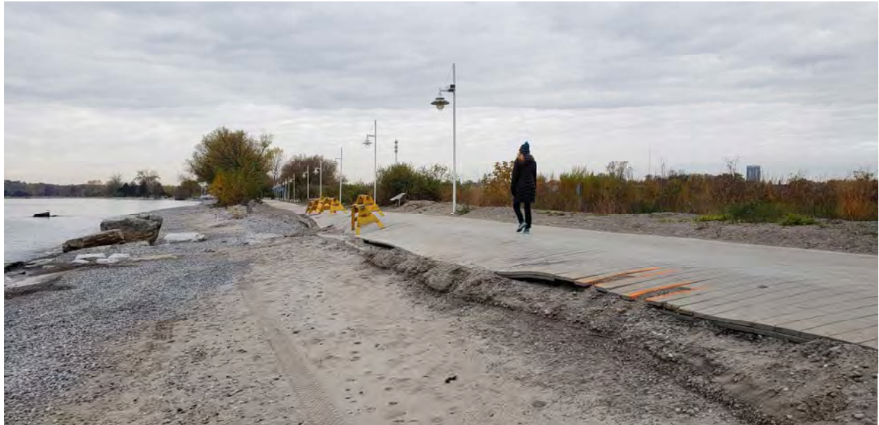
Figure 3: Beach erosion and damaged boardwalk near the east end of EBB2 on October 29, 2019. A city worker told Baird that the boardwalk was covered with 3~4 ft of sand after storm (date unknown). Sand was pushed back on the beach and subsequently taken away by waves. Few channels created in deposited sand back of the beach indicated overtopping water must have drained into Hydro Marsh.
