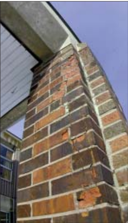
Some of the decay at Pickering High School is visible on this pillar out front of the school.
