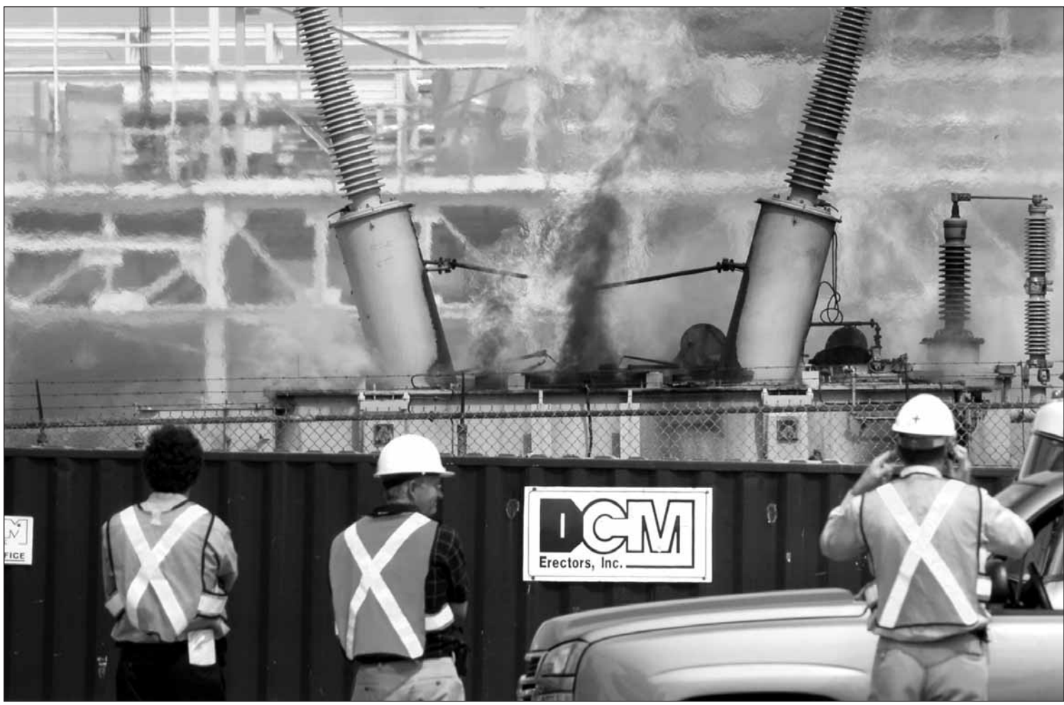
Flames rise at an electrical sub-station at the General Motors plant off Stevenson Road South in Oshawa.
