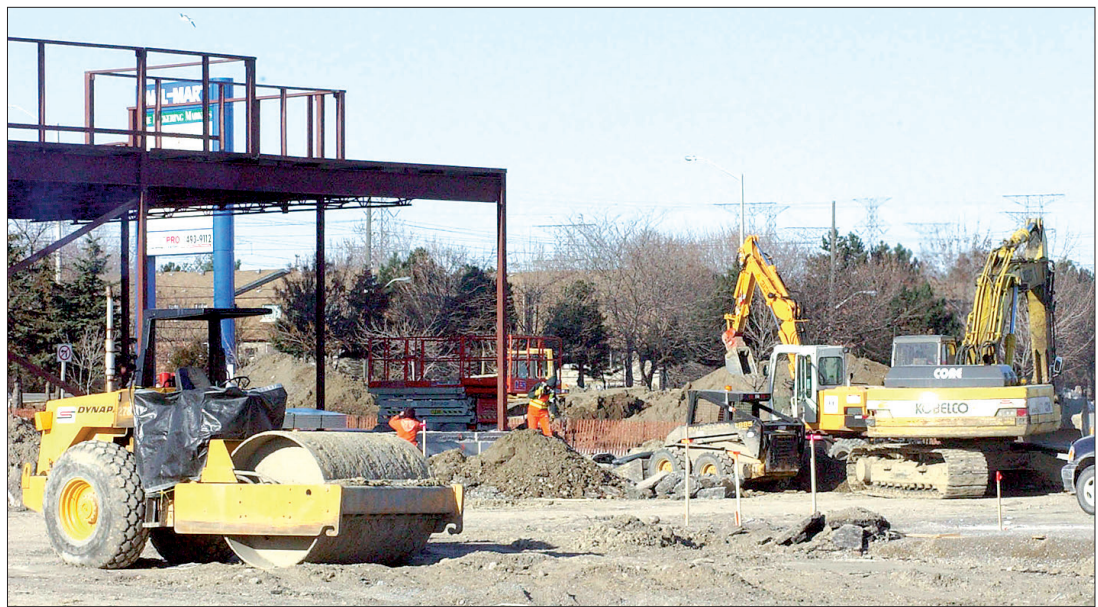
Construction is well under way on the Brock Road site between Hwy. 401 and Kingston Road. Several new stores are planned.
