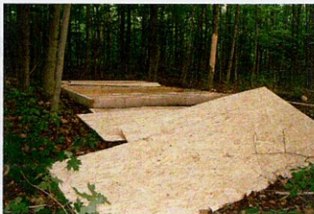
Drug house foundation with some of the building materials.
